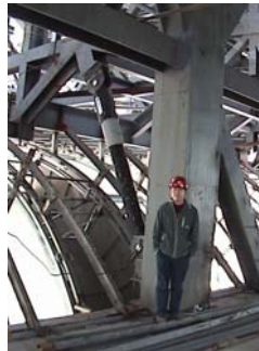
Fig.7 Installed 1500kN Damper
